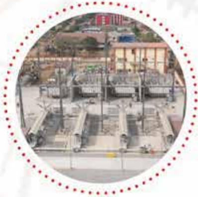
161kV Kasoa Bulk Supply Point (BSP), GRIDCo's 2nd largest Substation 2022
