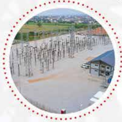
330kV Anwomaso Substation Kumasi, Ashanti Region, 2019
