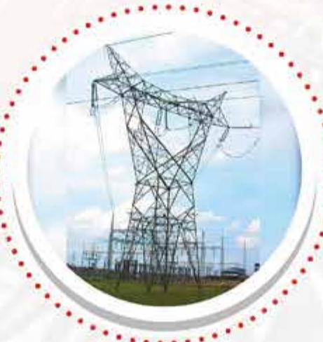
330kV Tower Volta Substation, Tema
