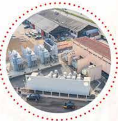
161kV Accra Central Bulk Supply Point (BSP) 2018
