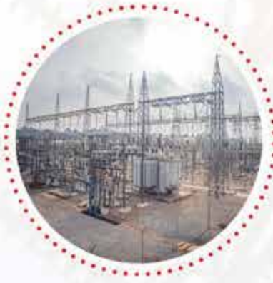
161kV Kumasi Substation, Ashanti Region, 1965
