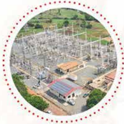
161kV Achimota Substation, Ghana's 1st Substation 1965
