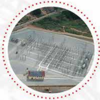
330kV Pokuase Bulk Supply Point (BSP), GRIDCo's Largest Substation, 2021
